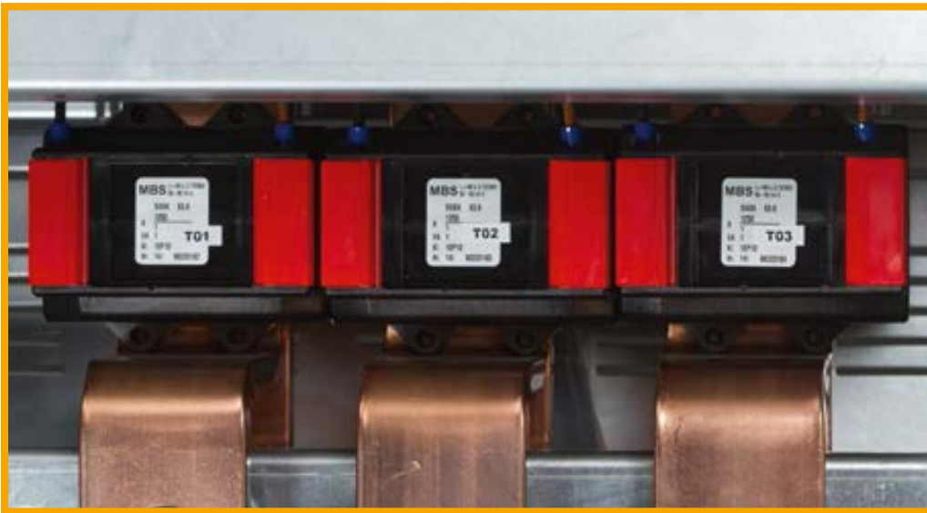
Fig. 9 Protection current transformer set
